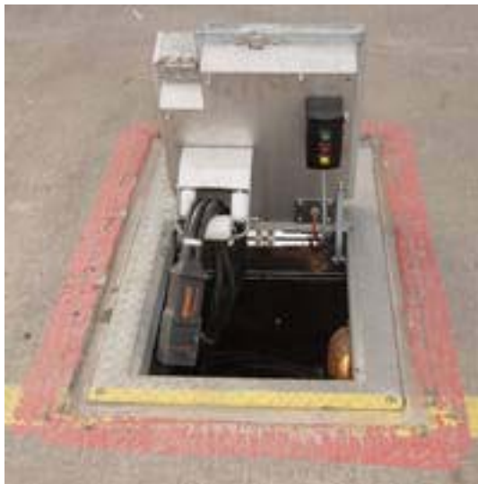
400Hz Power Pit
